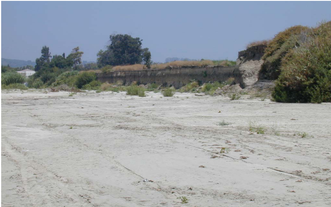
Calleguas Creek at Mission Oaks Blvd. (Bank Erosion), looking upstream
