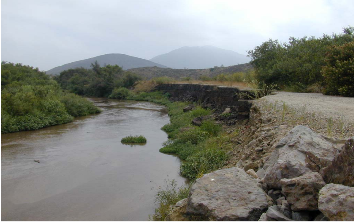
Calleguas Creek at Old Dairy Rd. (Erosion), near CSUCI, looking upstream
