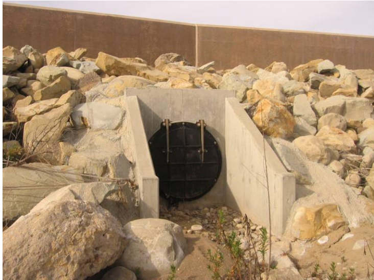
Ventura River Levee and Floodwall (Photo No. P1) – 48” RCP with a concrete outlet structure and Flap Gate
