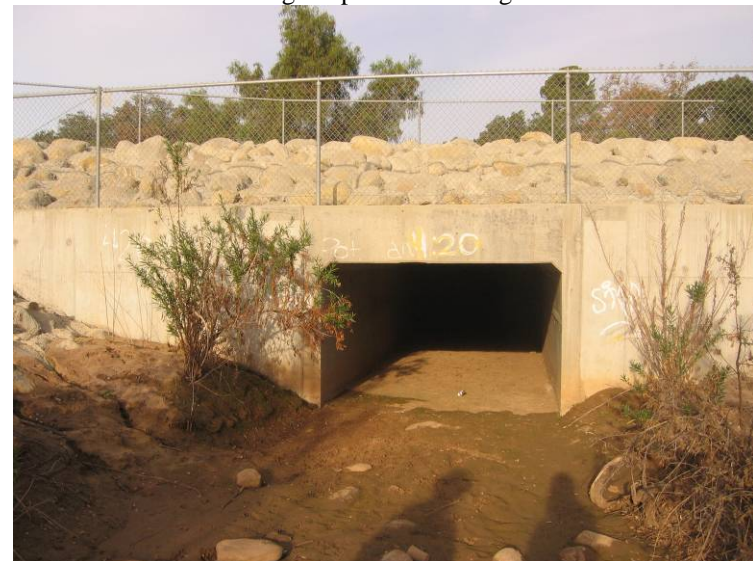
Ventura River Levee and Floodwall (Photo No. F2) – D/S face of 9’x5.6’ RCB outlet for the Live Oak Creek Diversion under Burnham Rd Bridge
