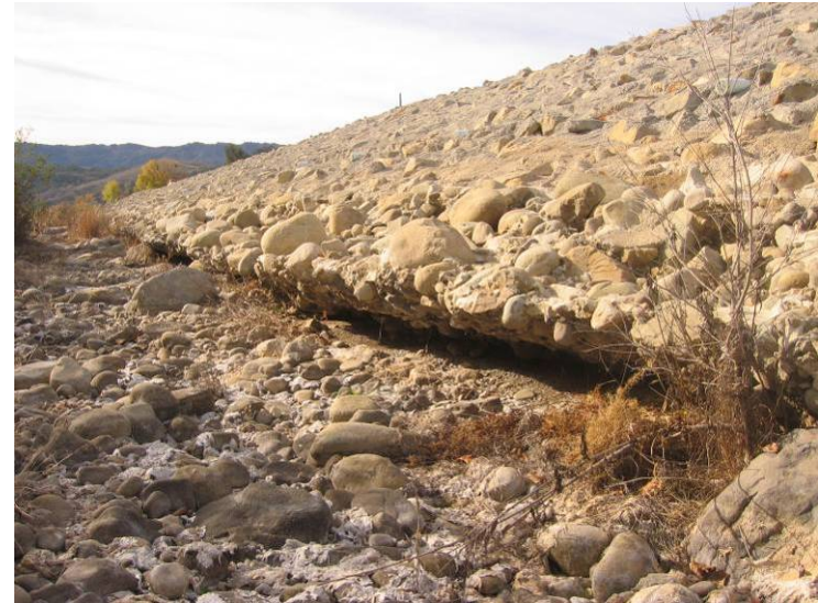
Ventura River Levee and Floodwall (Photo No. M3) – Erosion along levee toe below revetment (Riverward side)
