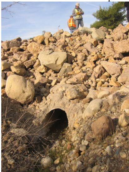
Ventura River Levee and Floodwall (Photo No. P2) – 24” CMP w/o a closure device
