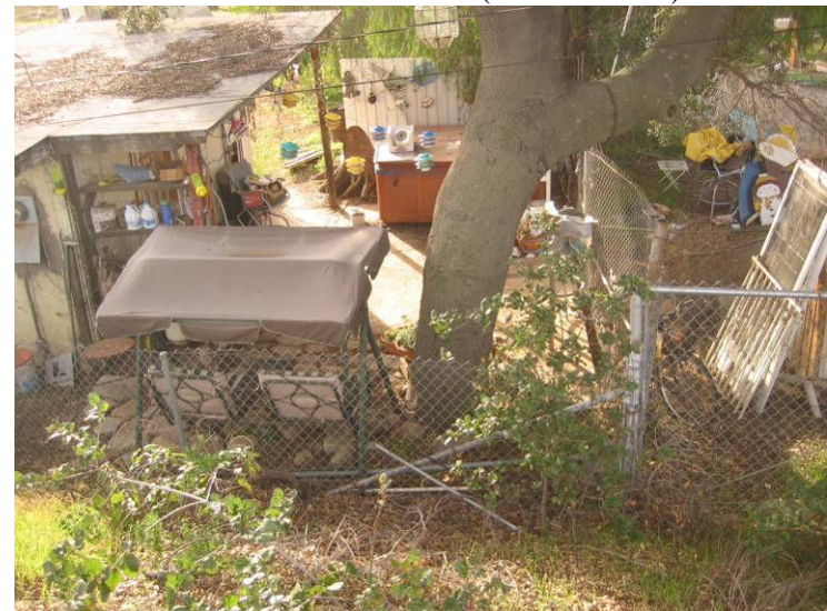
Ventura River Levee and Floodwall (Photo No. M4) – Encroachment. Structures within 15' of toe (Landward Side)
