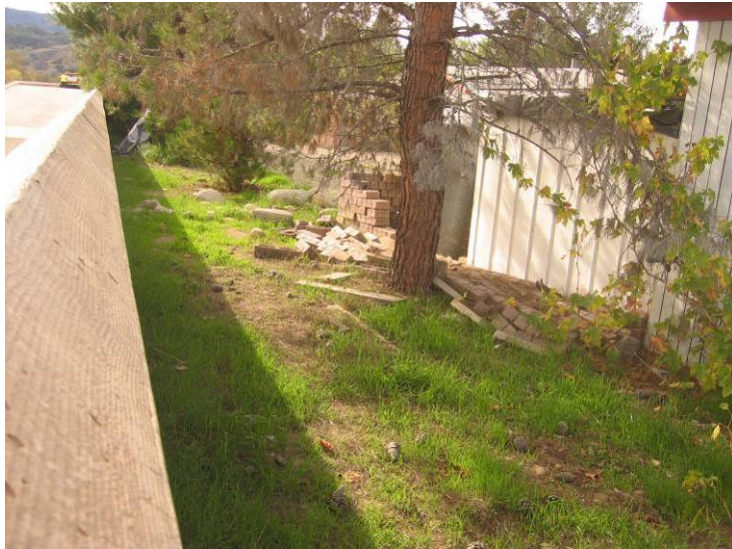
Ventura River Levee and Floodwall (Photo No. M1) – Vegetation within 15' of Toe (Landward Side)
