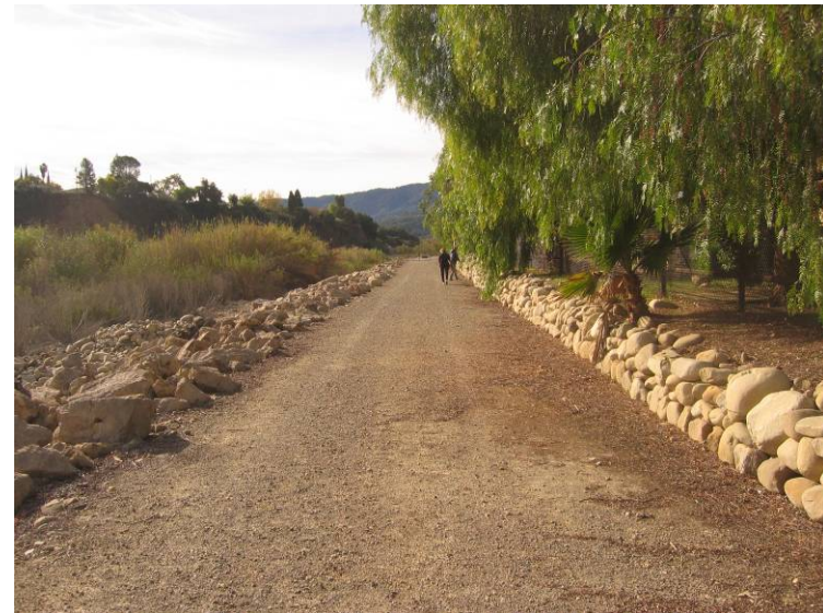
Ventura River Levee and Floodwall (Photo No. F1) – Looking downstream along a top of levee along Ventura River
