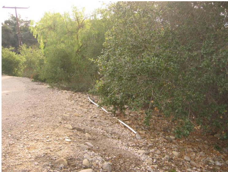
Ventura River Levee and Floodwall (Photo No. M5) – Vegetation within 15' of Toe (Landward Side)
