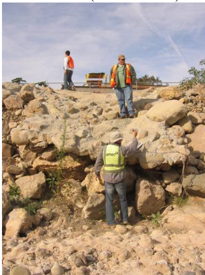
Ventura River Levee and Floodwall (Photo No. M2) – Undercut at the bottom of grouted stone apron of the levee top drain
