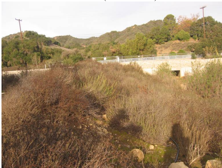
Ventura River Levee and Floodwall (Photo No. M6) – Vegetation on Levee embankment and toe (Riverward Side)
