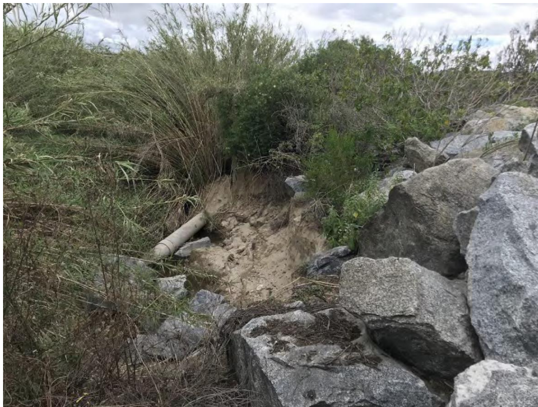
Figure 3-14: Damaged Sewer Pipe and Erosion
