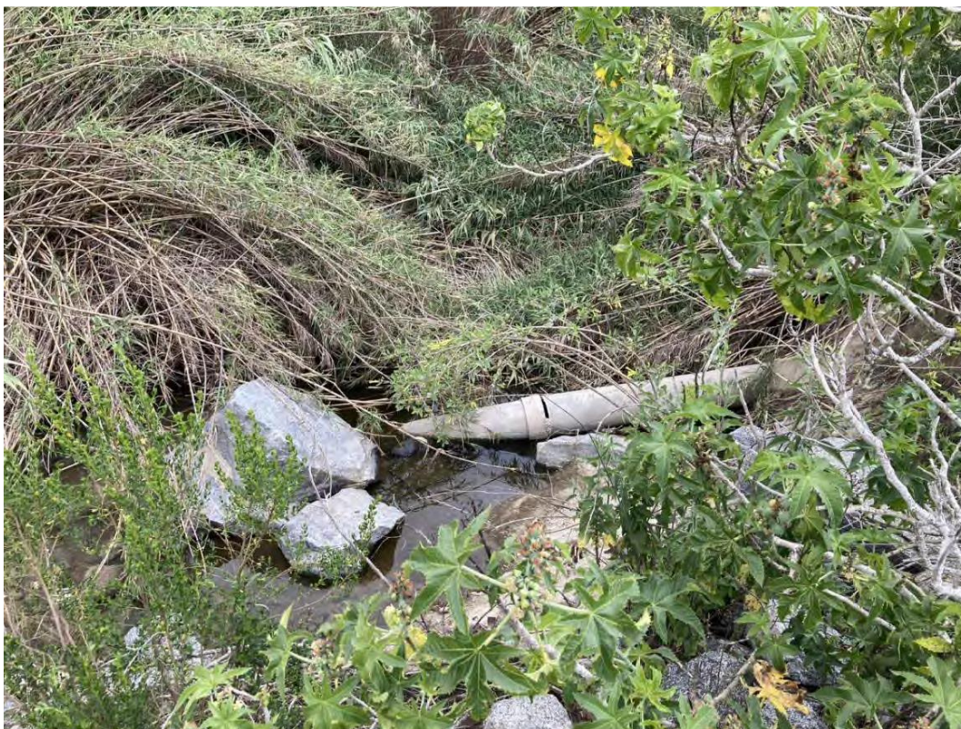
Figure 3-13: Broken 21" AC Sewer Piping
