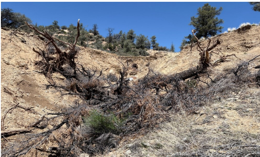
Photograph 12. View of CMP blowout in the southern portion of Unnamed Drainage 1 at MP 12.69, facing north (April 23, 2025).
