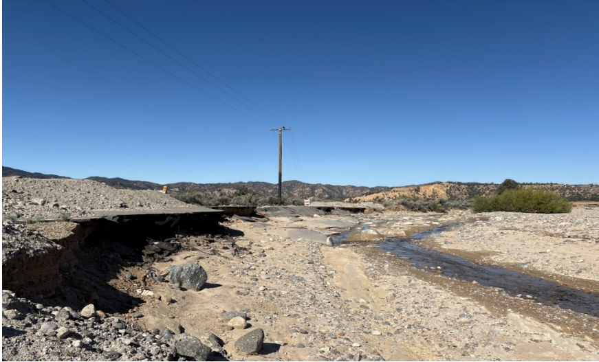
Photograph 1. View of the Cuyama River road washout on Lockwood Valley Road at MP 1.75, facing west (April 23, 2025).
