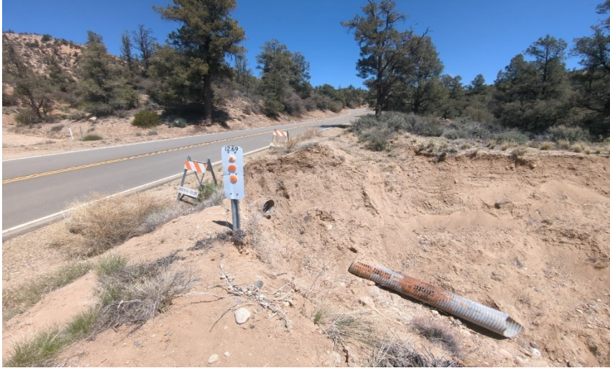
Photograph 13. View of CMP blowout in the southern portion of Unnamed Drainage 1 at MP 12.69, facing southeast (April 23, 2025).
