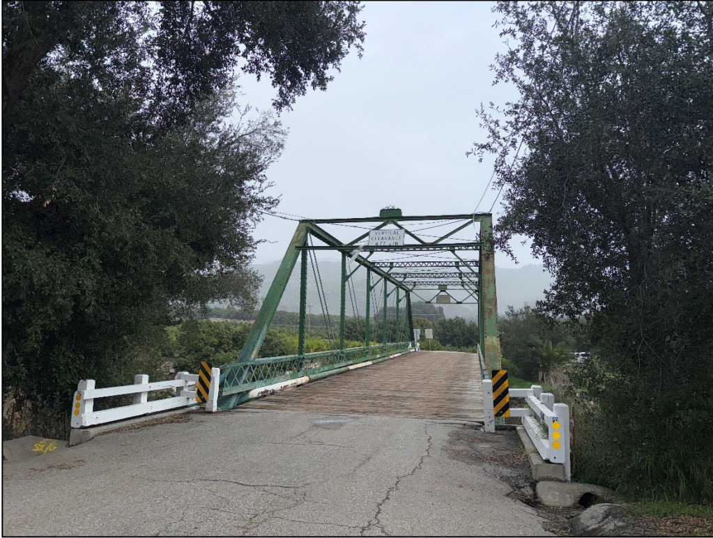
Photo 1. Bridge Road Bridge along the western edge of the Santa Paula Creek; view facing east. (January 2, 2026)
