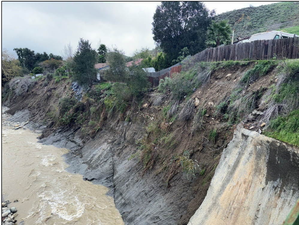
Photo 2. Santa Paula Creek south of Bridge Road Bridge, showing a severely eroded western bank; view facing south. (January 2, 2026)
