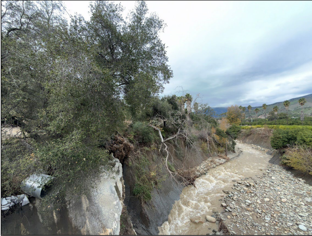
Photo 3. Santa Paula Creek north of Bridge Road Bridge, showing an eroded western bank, damaged concrete retaining wall, and coast live oaks ( Quercus agrifolia ); view facing north. (January 2, 2026)
